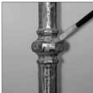
Application of the de-rusting product E4052/D: all polluted parts must be covered
